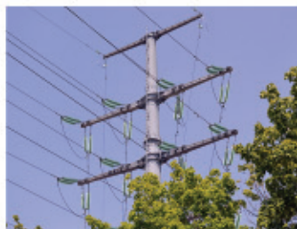
Power Line Clearance
